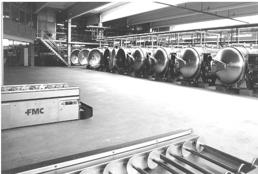
Fig. 1 Heat treatment plant with group of autoclaves (Simpson et al., 2007)
